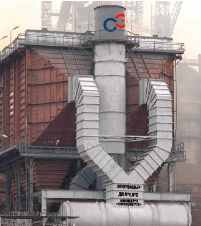
Electrostatic precipitator for cleaning aspiration emissions from foundries of blast furnaces.
